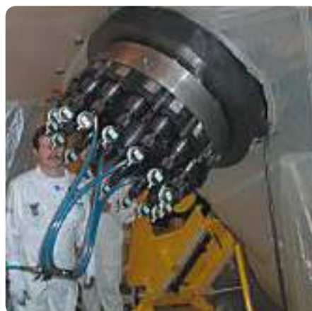
On-site intervention, tightening the man hole hatch on the primary cooling system of a steam generator
