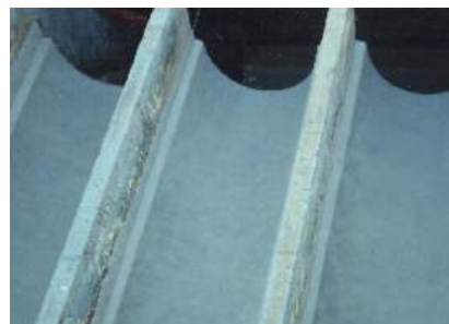
All three pump troughs coated with ARC 791
